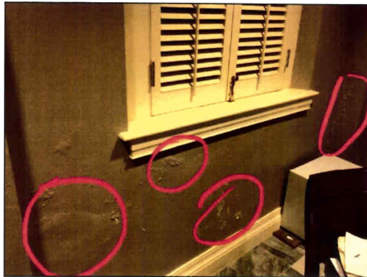
Figure 12: Detail of an Example of Interior Plaster Damage due to Water/Moisture Infiltration. Taken 11/7/2017.
