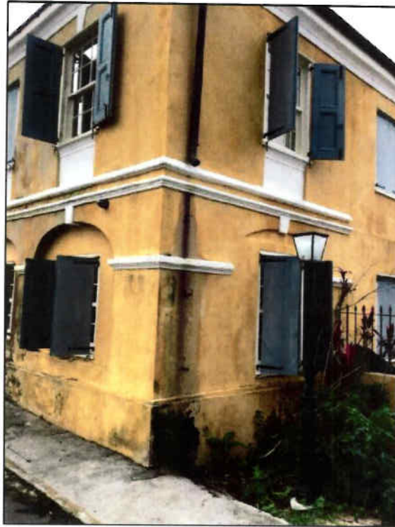
Figure 11: Danish School, Rear (East) and Side (North) Elevations, damaged gutter and wood panels. Taken 11/7/2017.
