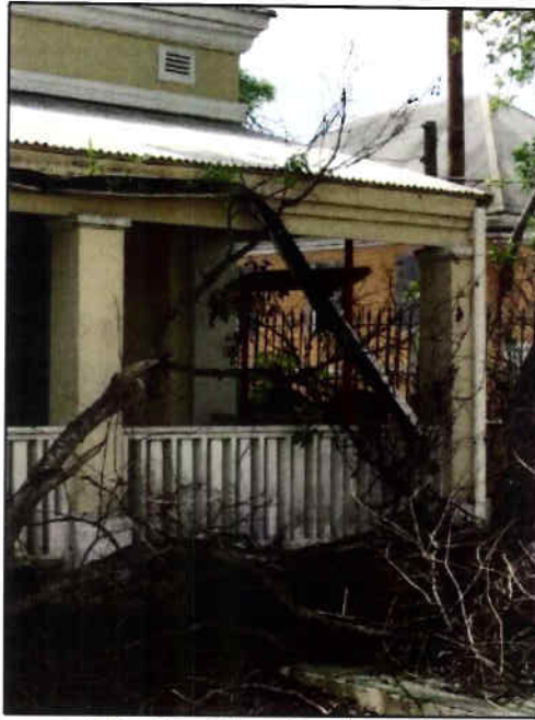
Figure 6: Annex Building, North Elevation, damaged gutter. Taken 11/7/2017.
