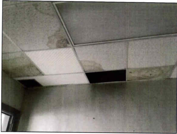
Figure 13: Detail of Multiple Roof Leaks in Annex Building, Exacerbated By Wind-Driven Rain, Looking West. Taken 11/7/2017.
