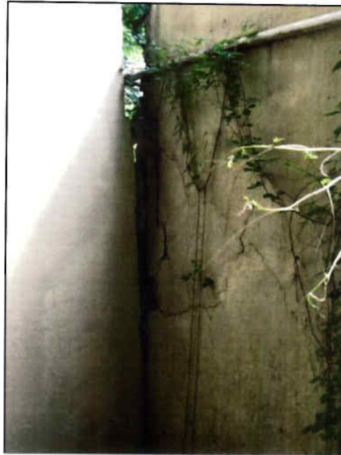
Figure 10: Detail of a Large Crack in the Annex Building's Breezeway Concrete Wall, Looking South. Taken 11/7/2017.
