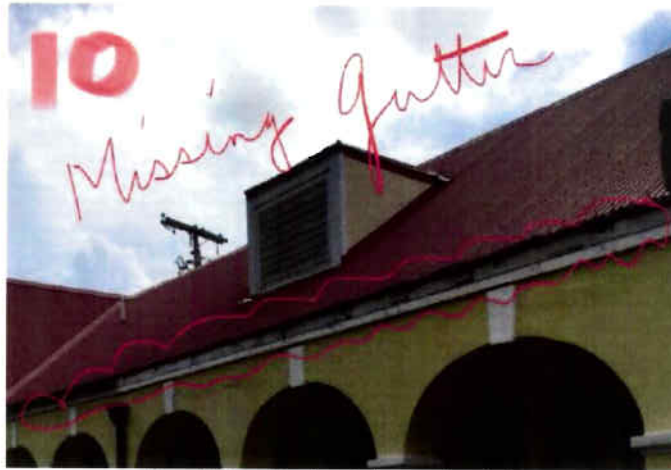
Description: Roof metal gutter is missing
