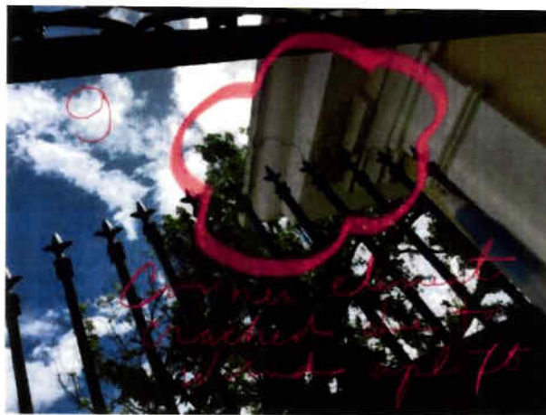
Description: Cracks and water damage along soffit cornice
