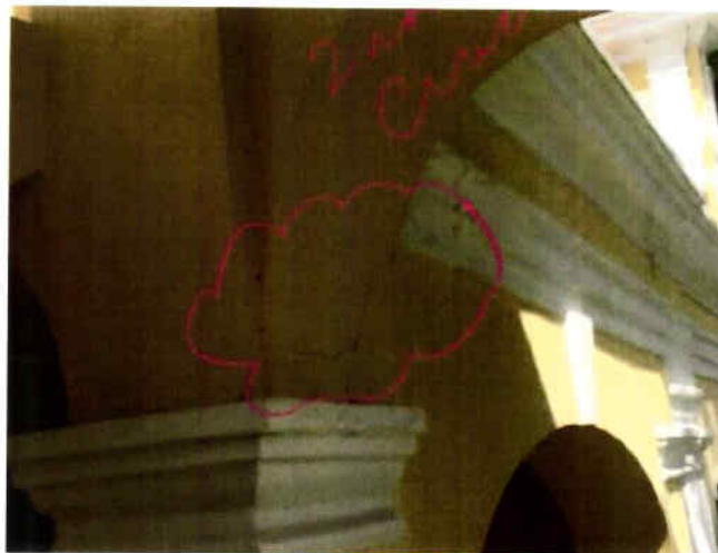
Description: Structural cracks in second floor arch
