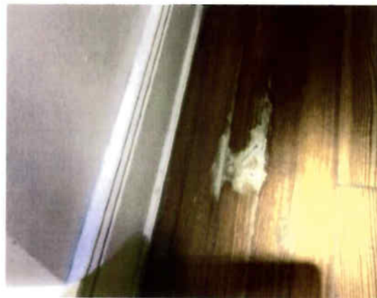
Description: Wood Flooring is water damaged
