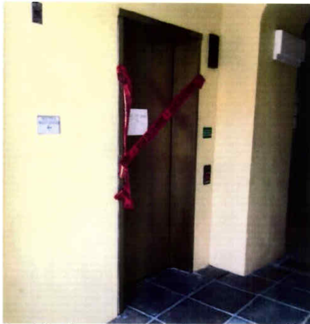
Description: Elevator not functioning due to water intrusion from above
