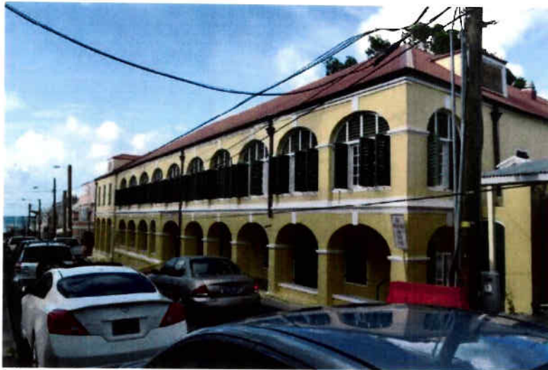
Sobotker portion of the building, with hipped roof, lower level gallery with arched openings and upper level with arched openings infilled with windows
