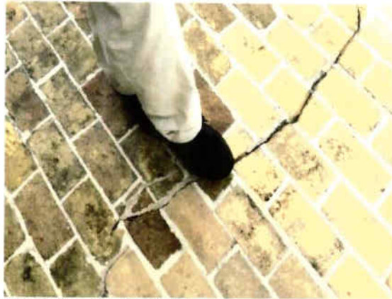
Description: Structural cracks along walkway
