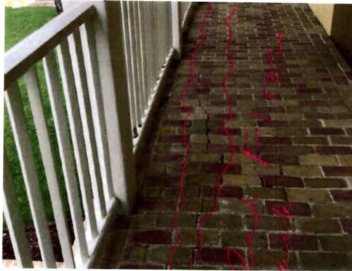
Description: Structural cracks along upper level of exterior corridor
