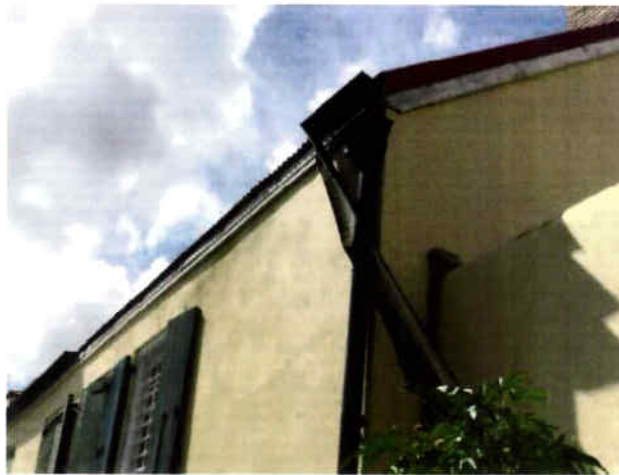
Description: Roof metal gutter is damaged
