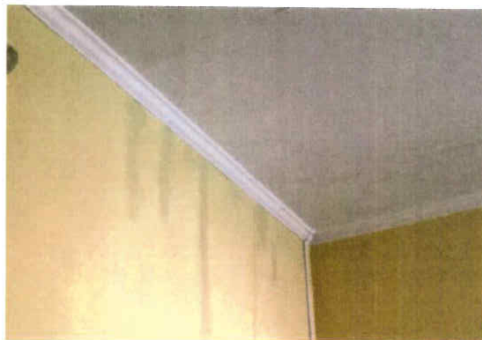
Description: Water damage at wall and ceiling due to water intrusion from above
