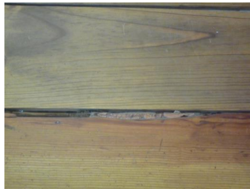
Item No. 07 Planters destroyed by tree roots
