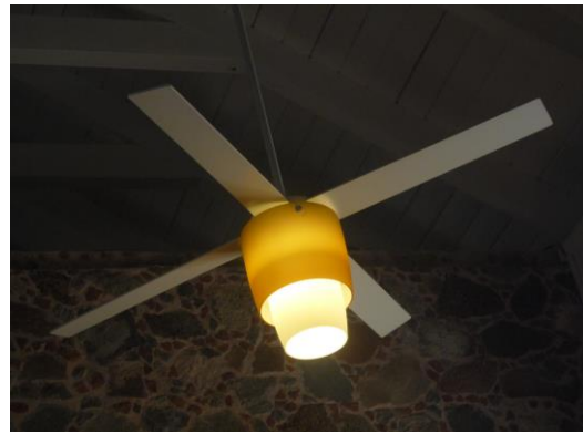
Item No. 02 light/fan to be repaired
