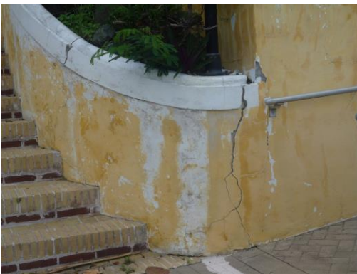
Item No. 06 Cracked stair masonry railing
