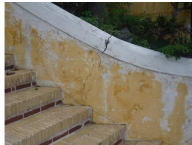
Item No. 04 Cracked stair masonry railing
