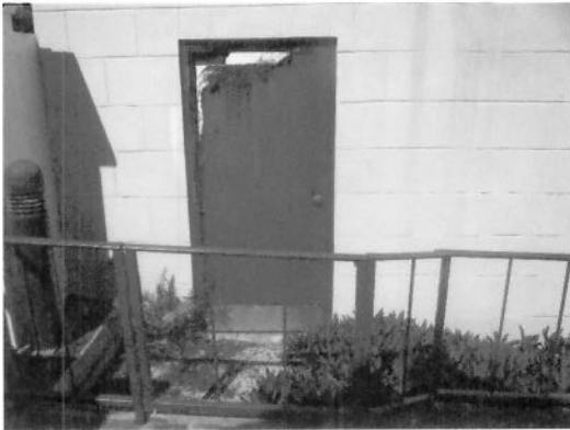
Item No. 1 metal door to be replaced
