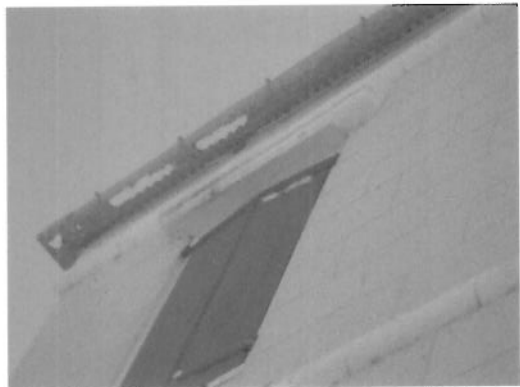
Item No. 46 Building's guttering to be replaced
