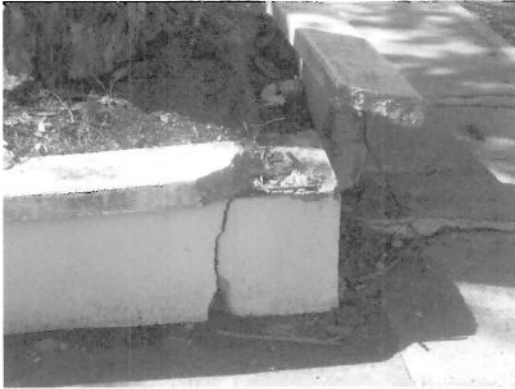
Item No. 50 Planters destroyed by tree roots
