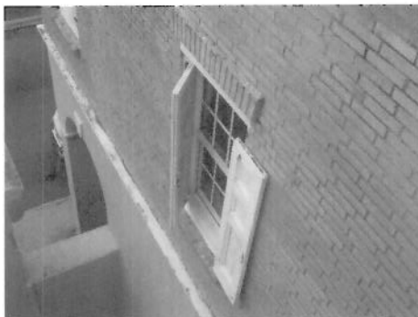
Bldg. Ledge to be sealed
